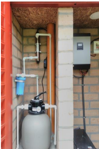
Figure 2. Rainwater harvesting and treatment system
