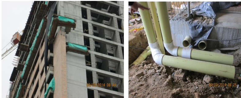
Figure 1. Double pipe for rainwater harvesting at height.
